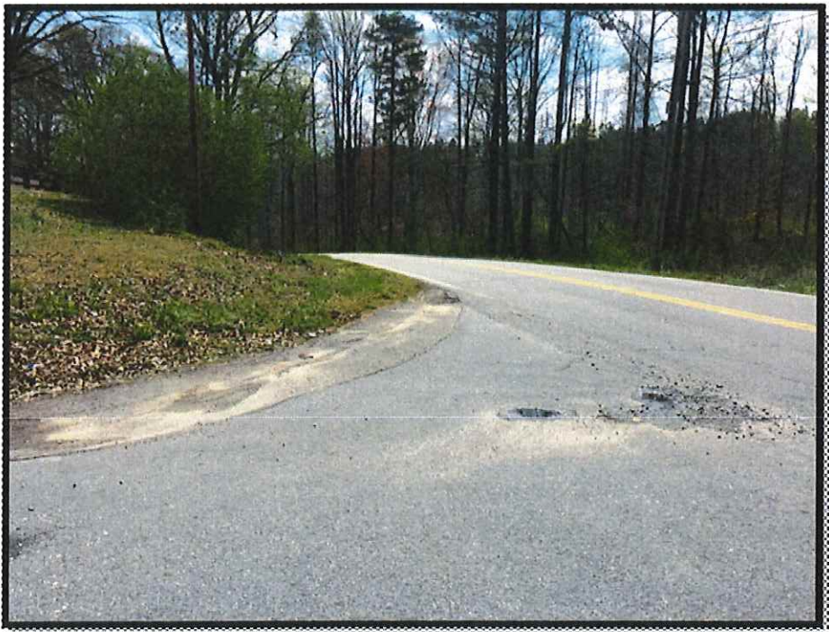
Photograph 5 – View From Driver's Eye on Southbound Grimes Road Facing East at Arnold Mill Road
